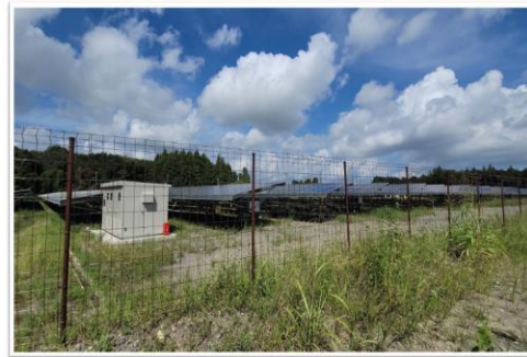
↑ Kami Ishikawa Solar Power Plant
