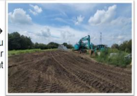
→ Site of Nasu Karasuyama Solar Power Plant
